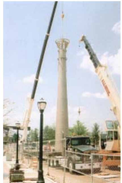
The telecommunications tower in Atlanta.
